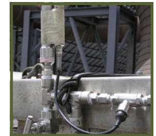
Orifice Plate Monitoring
